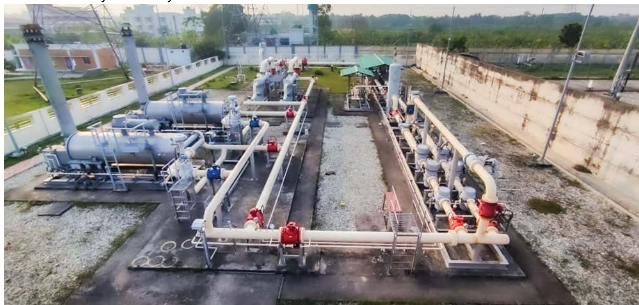
North-West Power Generation Company Limited’s 410 MW CCPP RMS, Bheramara, Kushtia under SGCL
