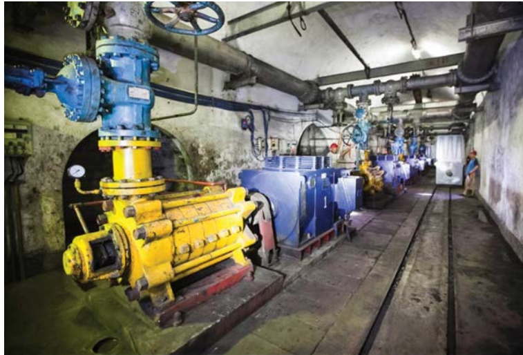
Underground Pump House at (-260) m level of BCMCL
