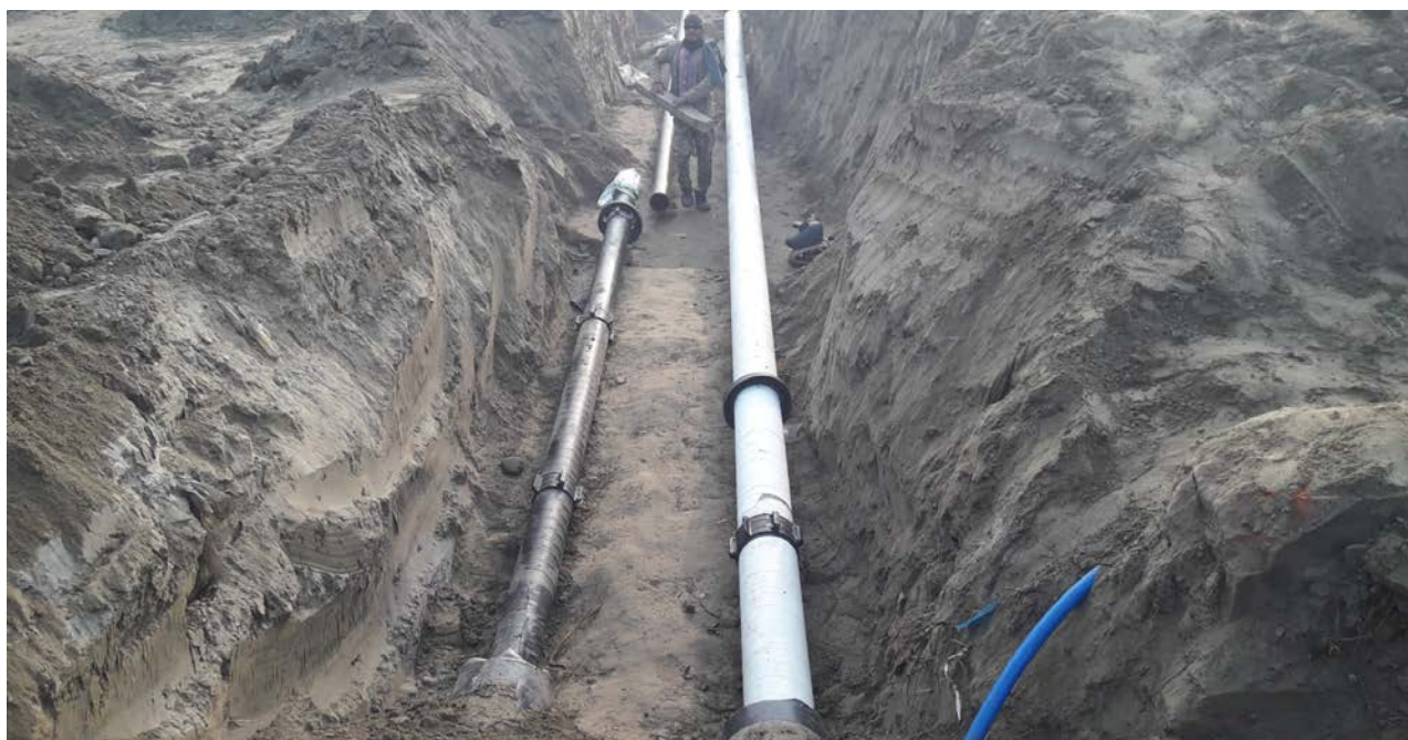
SASEC-2 Depository Funded Pipeline Construction (Major Road Crossing) Work at Nalka by PGCL.
