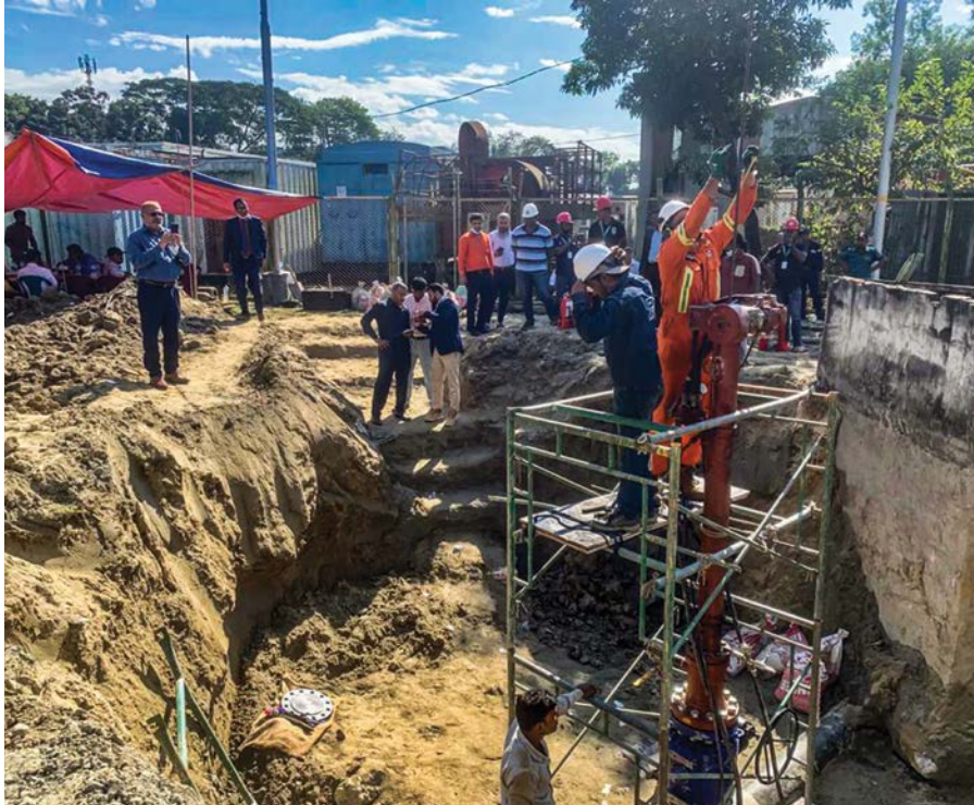
12" dia to 8" dia pipeline hot tapping works at GTCL valve station, Madhabpur by JGTDSL.
