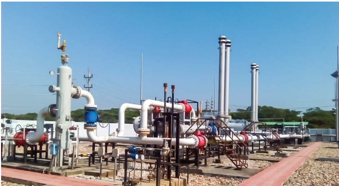
PDB's 225 MW CCPP RMS, Borhanuddin, Bhola under SGCL
