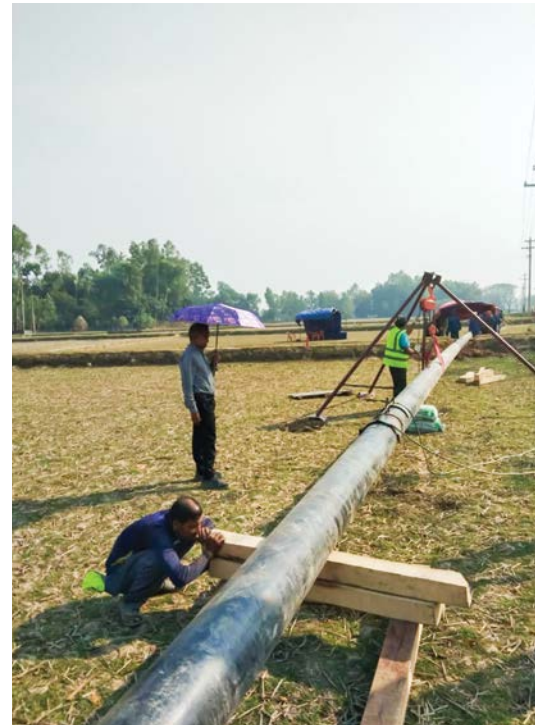
Construction works of 10" dia x 300 PSIG x 17 Km pipeline from Mirpur Natun Bazar DRS to Putijuri Bahubol, Habiganj by JGTDSL
